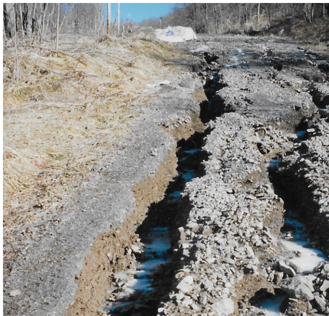
18" ruts in Skyline Lakes roads after Nor-easter of 1996
